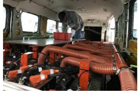
Fig. 10 Battery Cluster Assembly, Ducting, & False Floor
