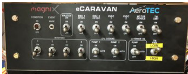
DAS Rack Switches
