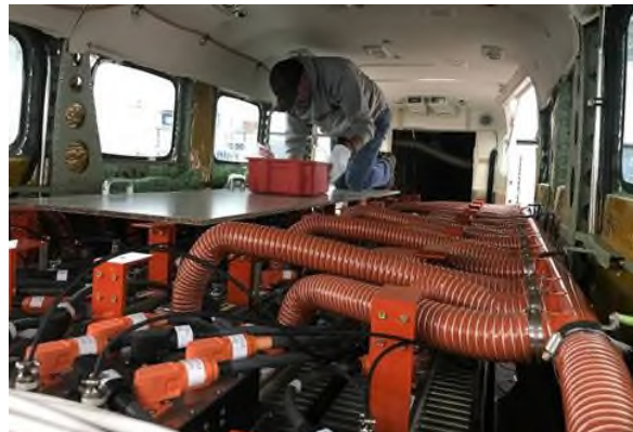
Fig. 10 Battery Cluster Assembly, Ducting, & False Floor
