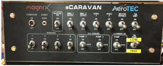
DAS Rack Switches
