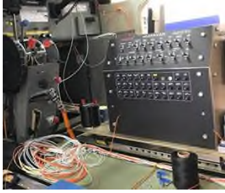
DAS Rack & Mounting Plate on Co-pilot's Seat Rails
