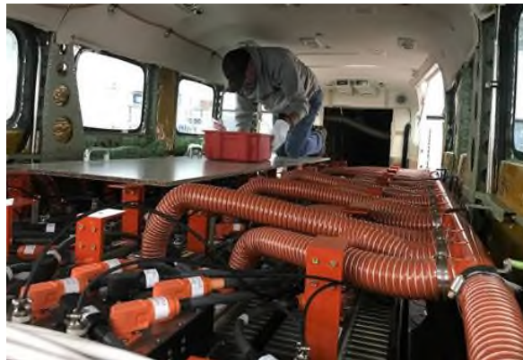
Figure 10 – Battery Cluster Assembly, Ducting, & False Floor
